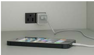
Interior Power Outlet
